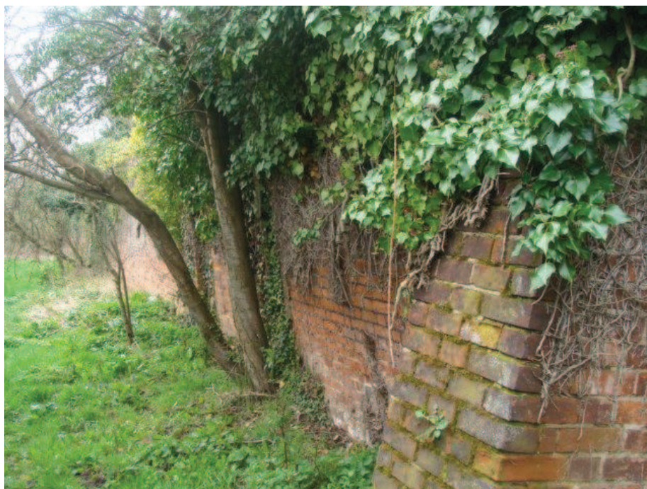
Picture 23 - Detail of fine walls to walled garden historically associated with Danes. They are generally in good condition but would benefit from removal of selected vegetation in some locations such as ivy that may be causing damage.
